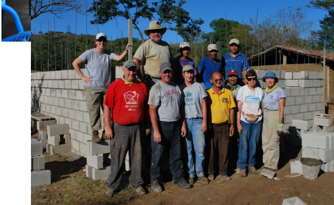
Part of our team pictured with the masons in front of one of the houses we helped start from the ground up (below)
